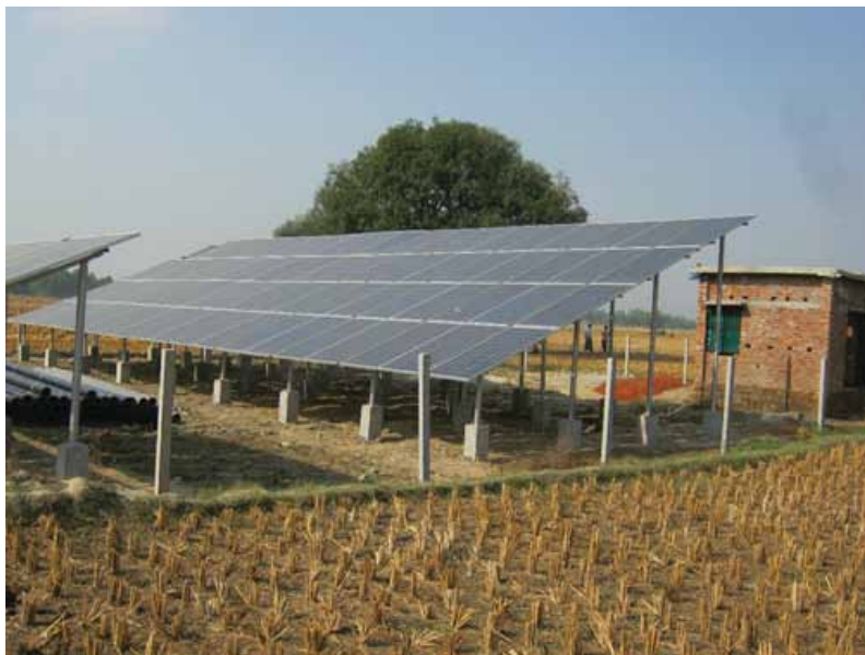
Solar Irrigation Pump
