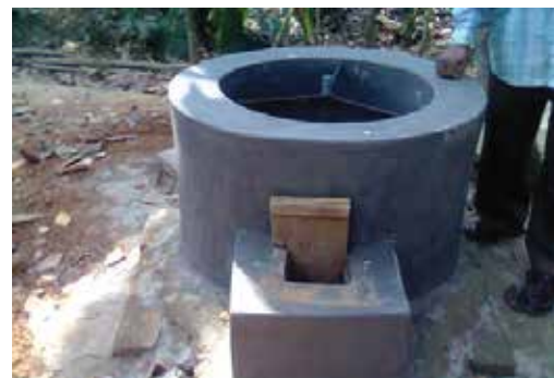
Mixing Device of Biogas plant
